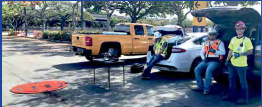
Hensel Phelps sUAS team receives flight clearance from DKI International Airport's tower for HP's Mauka Concourse project.
