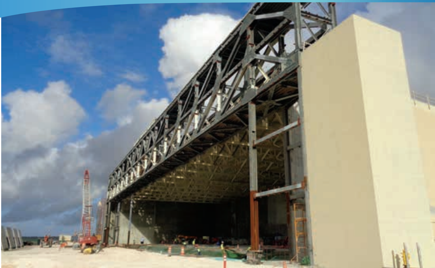
NAVFAC's P-109 Aircraft Maintenance Hangar during construction, a recent Guam project by Baldrige & Associates Structural Engineering Inc. PHOTO COURTESY BASE
