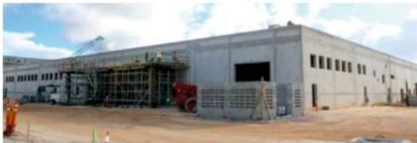
Black Construction's P-250 MALS project, combined with the P-260 Corrosion Control Hangar project, is valued at $86 million.
